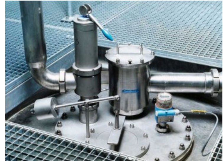
CO 2 -head pressure measurement at the fermentation tank with Deltapilot S DB50L
