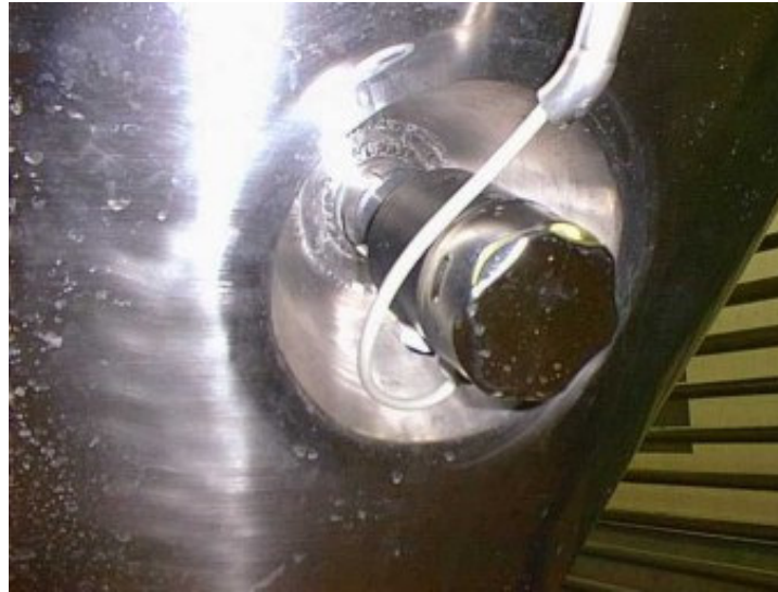
Level measurement at the fermentation tank in the brewery with Deltapilot S DB50L
